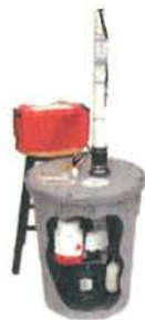
Pump with ultrasump battery back up pumping system
