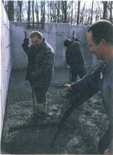
The less slump to the concrete, the less shrinkage cracking and higher compressive strength. The aggregate bed under the floor provides a good base and drainage under the slab. A vapor barrier is beneath the aggregate.
